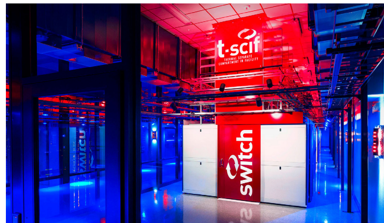
Photo courtesy of Switch
