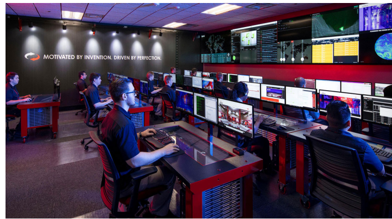
Photo courtesy of Switch
